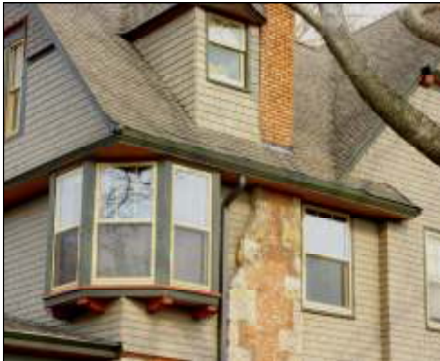
My rebuilt box gutters I have had the privilege of Bill's workmanship on my own Hyde Park residence. Here he rebuilt my box gutters and did numerous woodwork repairs.
